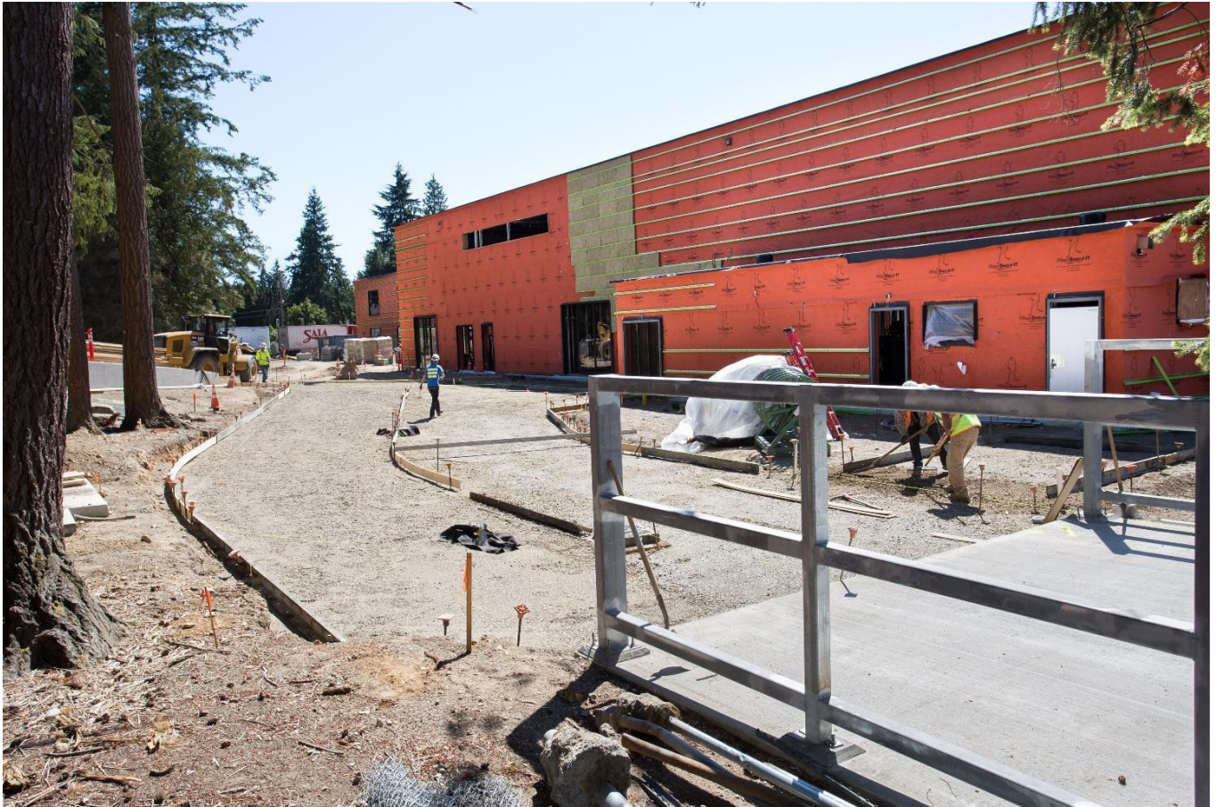
Construction of Lynndale Elementary School in Edmonds School District. (Photo Credit: Legislative Support Services)
